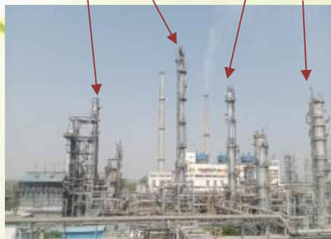
Vent Silencer in Ammonia-I Plant
