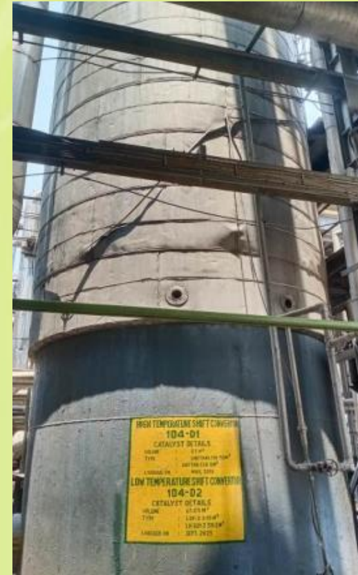
View of LTS Converter
